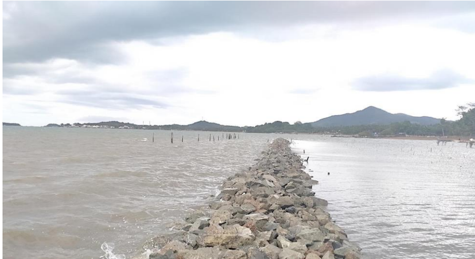
Figure 12. The breakwater reduces wave energy before it hits the shore and provides protection to the mangrove rehabilitation area and coastal communities.
